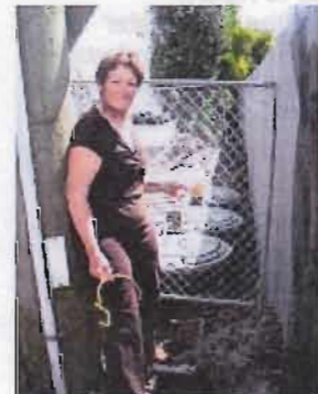
Carol with the newly installed grinder pumps outside her property on Park Road
